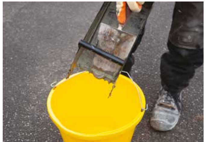
4. Remove any remaining ZeroPlus mortar from the trough before thoroughly washing that out also.
