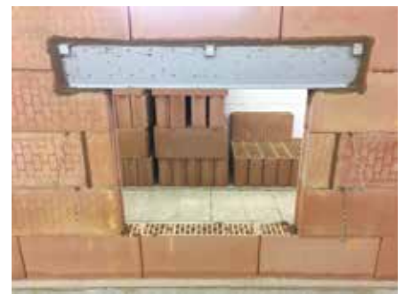
3. The lintel can then be built in using traditional mortar and again using boot cuts where possible.
